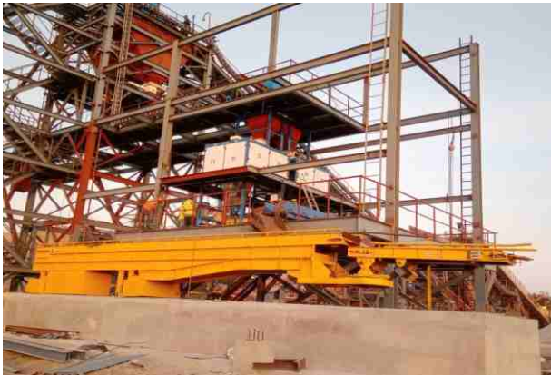
VT Corp's Truck Loader installed at JSW Steel Plant
